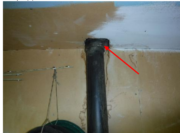
Photo 6 Description: Bell and spigot pipe gaskets
