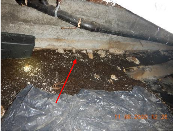
Photo 5 Description: Pipe insulation debris remnants
