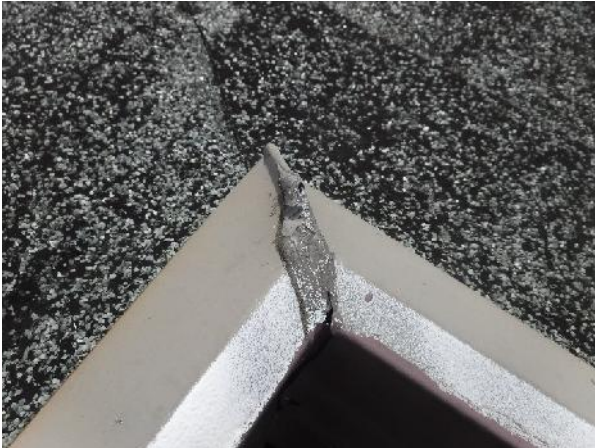
Photo 1 Description: Mastic (Black/Grey) Location: Roof Flashing Asbestos: 7% chrysotile Sample(s): 39956-8b
