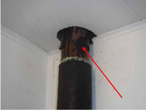
Photo 5 Description: Pipe mastic – black Location: Janitors Closet Asbestos: Suspect
