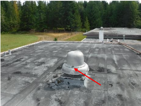
Photo 3 Description: Mastic (Black with white specks) Location: Roof Asbestos: 9% chrysotile Sample(s): 39956-14b
