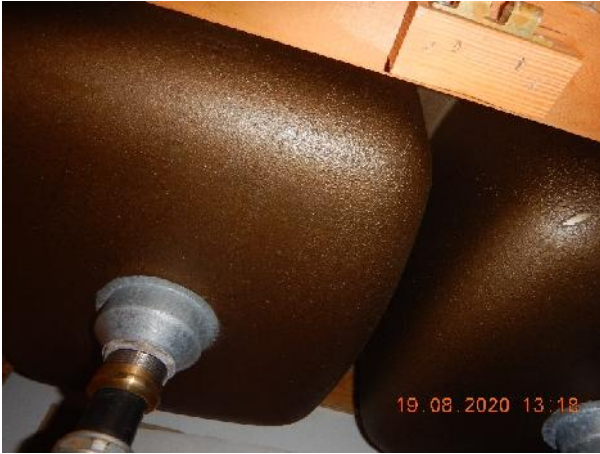
Photo 5 Description: Acoustic sink insulation – black/silver Location: Kitchen Off Gym Asbestos: Suspect
