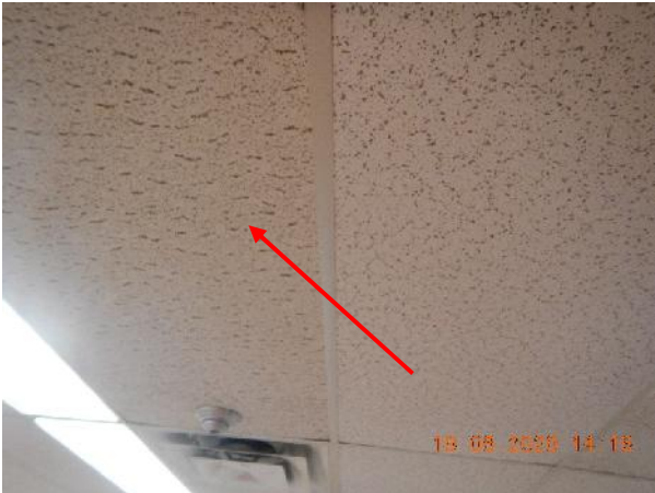
Photo 5 Description: Acoustic ceiling tile 2 – latitudinal fissures, small and large pinholes Location: Mezzanine Boys Dressing Room and Washroom Asbestos: Suspect
