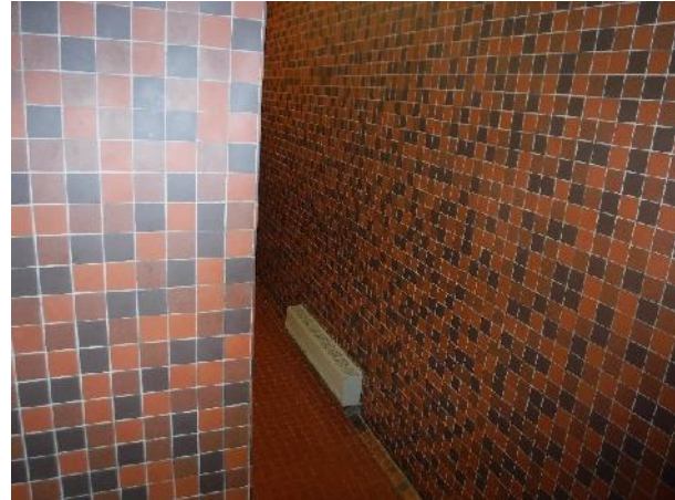
Photo 6 Description: 1.5" red and brown ceramic tile grout Location: Boys Washroom By Room 302 Asbestos: Suspect
