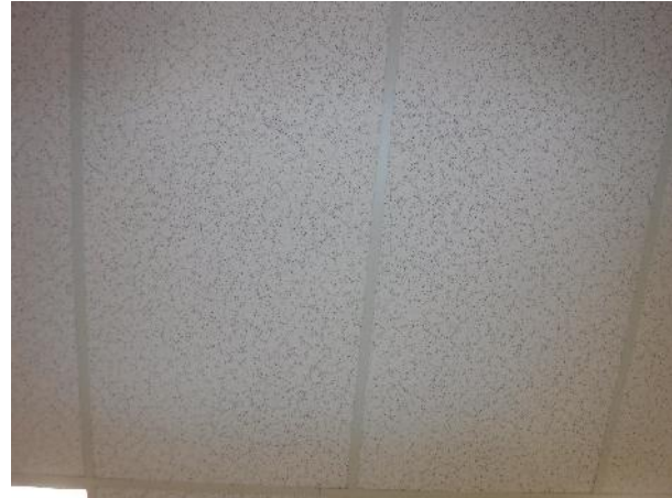
Photo 6 Description: Acoustic ceiling tile 1 – patterned fissures, small and large pinholes Location: Room 301 Asbestos: Suspect
