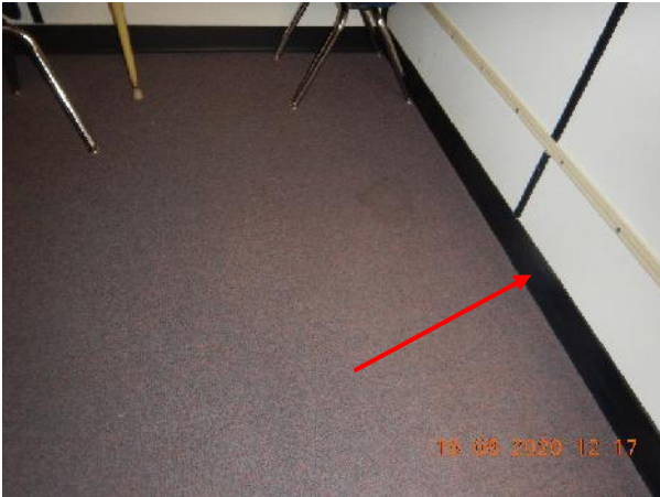
Photo 5 Description: Baseboard adhesive Location: Throughout Asbestos: Suspect
