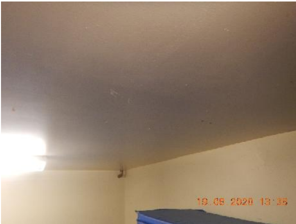
Photo 1 Description: Drywall Joint Compound Location: Stage Storage Room off Gym Asbestos: 1.7% chrysotile Sample(s): 30013-3
