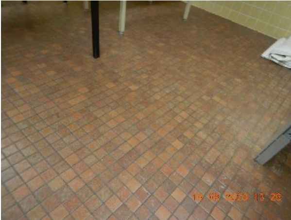
Photo 5 Description: 2"x2" brown ceramic tile grout Location: Girls Change Room Off Gym Asbestos: Suspect
