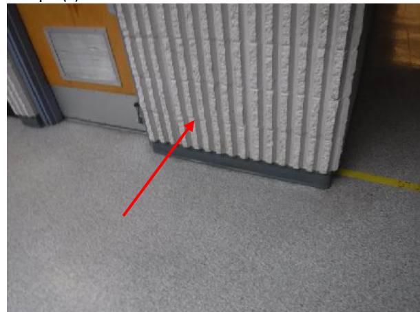
Photo 4 Description: Concrete block (may contain vermiculite) Location: Hallway by Room 304 Asbestos: Suspect
