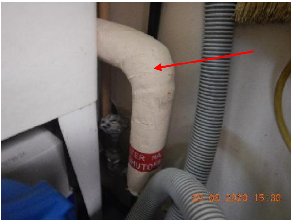
Photo 11 Description: Cementitious pipe elbow Location: Lower Level – Custodian Room Asbestos: Suspect
