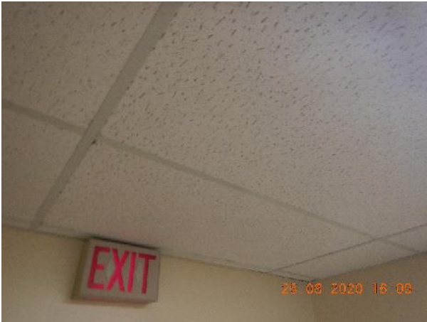
Photo 7 Description: Acoustic ceiling tile 2 – lateral fissure Location: Lower Level – West Exit Asbestos: Suspect
