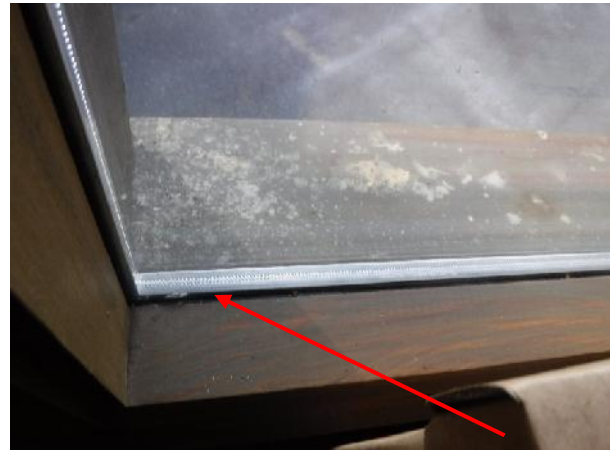
Photo 2 Description: Window putty – black Location: Room 111 – Secretary First Nation Asbestos: 12 % Chrysotile Sample(s): 39957-47b
