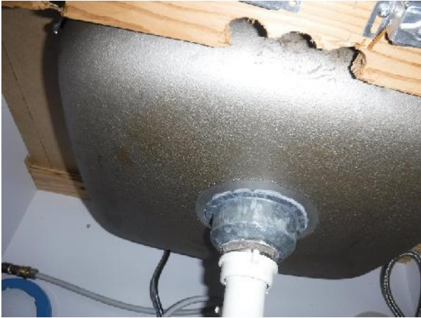
Photo 5 Description: Acoustic sink insulation – gold/silver Location: Room 117 Asbestos: Suspect
