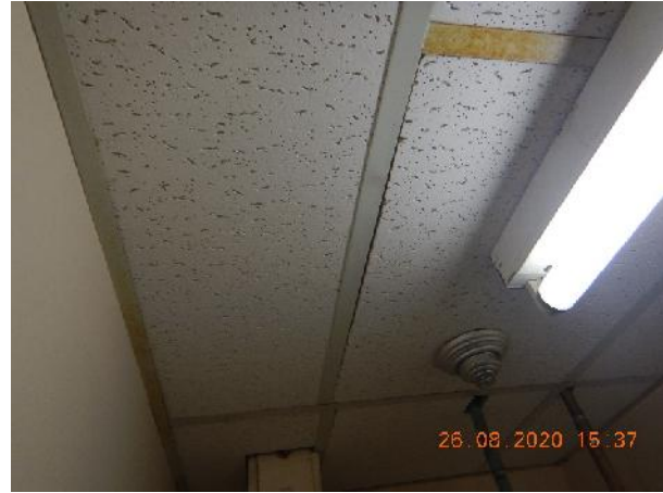
Photo 6 Description: Acoustic ceiling tile 1 – small and large pinhole Location: Lower Level – Custodian Room Asbestos: Suspect
