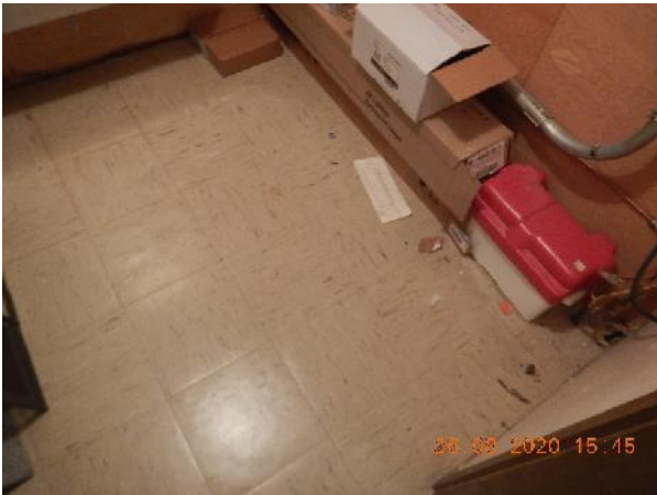
Photo 1 Description: Floor tile 1 – 12”x12” brown with white streaks Location: Lower Level – Electrical Room Asbestos: 2.4% Chrysotile Sample(s): 30011-8
