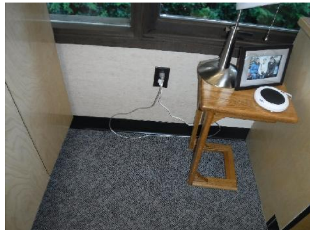
Photo 12 Description: Baseboard adhesive Location: Room 116 – Superintendent of Schools Asbestos: Suspect
