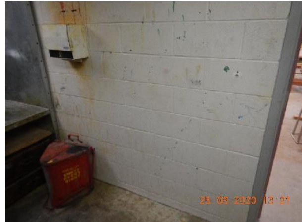
Photo 2 Description: Concrete block (contains vermiculite) Location: Room 607 Asbestos: 0.5%Tremolite Sample(s): 31788-22
