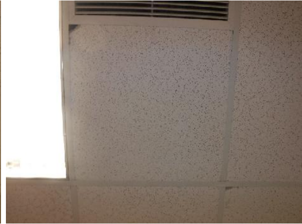
Photo 6 Description: Acoustic ceiling tile 3 – patterned fissure small and large pinhole Location: Asbestos: Suspect
