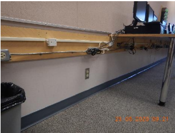
Photo 27 Description: Baseboard adhesive Location: Room 355 Asbestos: Suspect
