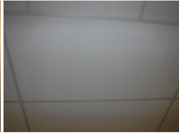
Photo 8 Description: Acoustic ceiling tile 5 – pinhole Location: Hallway 1 Asbestos: Suspect
