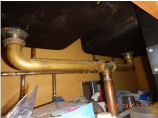
Photo 1 Description: Sink mastic – black Location: Room 507 Asbestos: 6.8%chrysotile Sample(s): 30009-20
