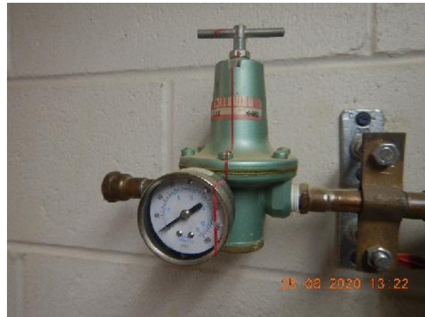
Photo 28 Description: Gasket Location: Room 607 Asbestos: Suspect
