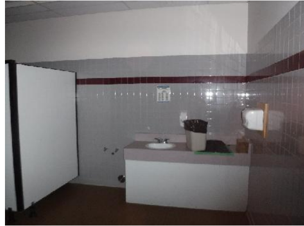
Photo 10 Description: Ceramic tile – 4"x4" grey Location: Men's Washroom Off Hallway 5 Asbestos: Suspect
