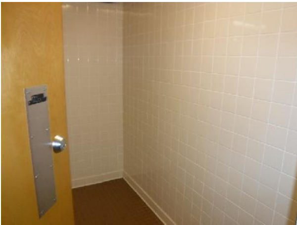
Photo 11 Description: Ceramic tile – 4"x4" white Location: Women's Change Room Asbestos: Suspect
