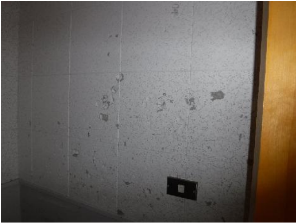
Photo 7 Description: Acoustic ceiling tile 4 – 1'x1' pinhole with random fissure Location: Room 132 Asbestos: Suspect
