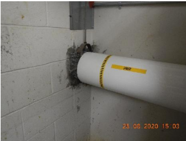
Photo 19 Description: Firestop – grey Location: 645 Mezzanine Boiler Room Asbestos: Suspect
