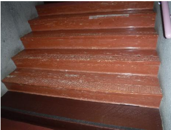
Photo 15 Description: Stair tread – red Location: Stairwell off Gym to Mezzanine Asbestos: Suspect
