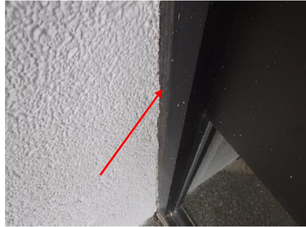
Photo 18 Description: Caulking – brown Location: Exterior Asbestos: Suspect
