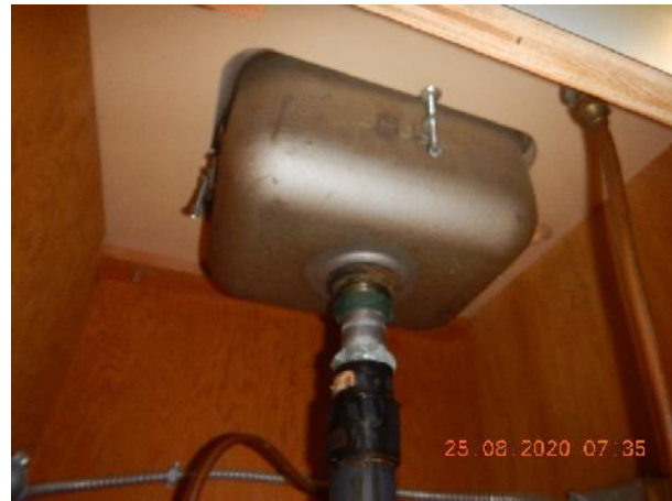
Photo 24 Description: Sink mastic – gold/silver Location: Room 300 Asbestos: Suspect
