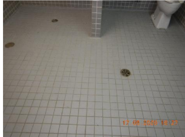
Photo 24 Description: 4"x4" grey ceramic tile grout and mortar Location: Handicap Washroom by Main Office
