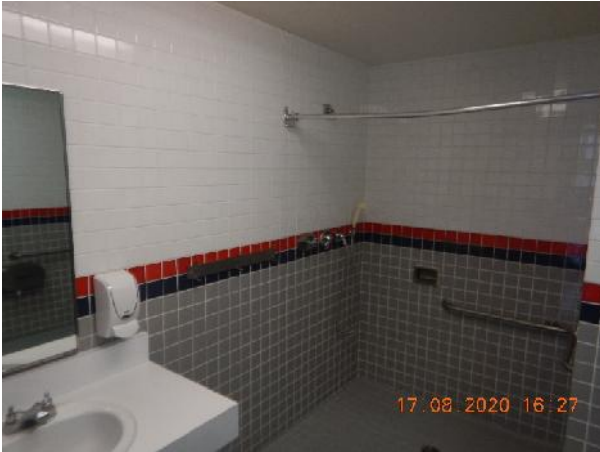
Photo 23 Description: 4"x4" white, grey, red and black ceramic tile grout and mortar Location: Handicap Washroom by Main Office
