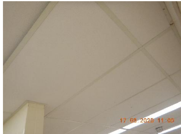
Photo 18 Description: Acoustic ceiling tile 5 – Textured fibreglass Location: Hallway 4 Gentlemen Washroom Asbestos: Suspect
