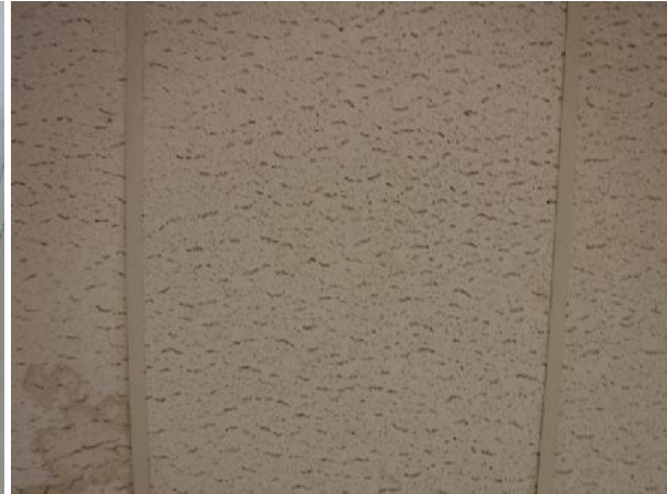
Photo 16 Description: Acoustic ceiling tile 3 – Vertical fissure small and large pinholes Location: Asbestos: Suspect
