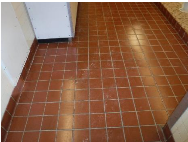
Photo 25 Description: 6"x6" red ceramic tile grout and mortar Location: Boys Washroom off Hallway 3
