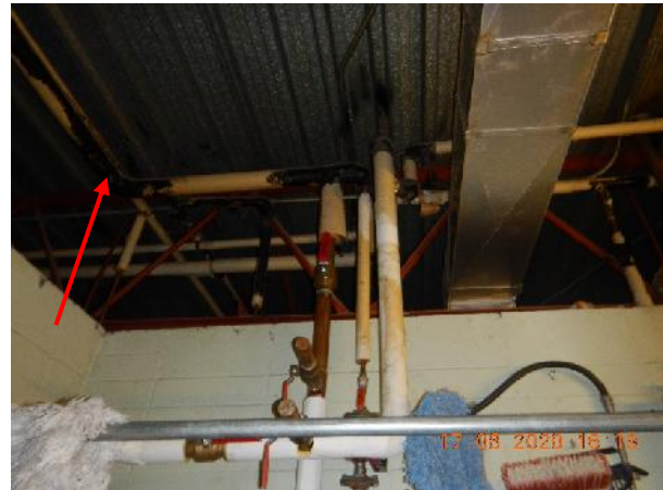
Photo 10 Description: Mastic 1 – Black on pipe insulation Location: Hallway 8 Janitors Room Asbestos: Suspect
