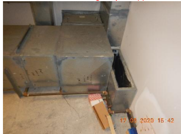
Photo 14 Description: Caulking 4 – Grey/white (Likely originally grey but painted white) Location: Mechanical Room Adjacent Drama Asbestos: 3.8% Chrysotile Sample: 30007-6
