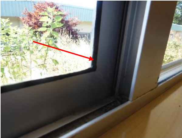
Photo 3 Description: Caulking 5 – Black Location: Room 227 Asbestos: 9% Chrysotile Sample(s): 40391-17b
