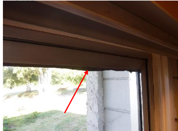
Photo 4 Description: Caulking 6 – Grey Location: First Nations Room Asbestos: 12% Chrysotile Sample(s): 40391-29b
