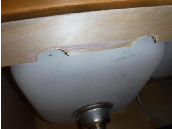
Photo 11 Description: Mastic 4 – White on sink Location: Room 227 Asbestos: Suspect
