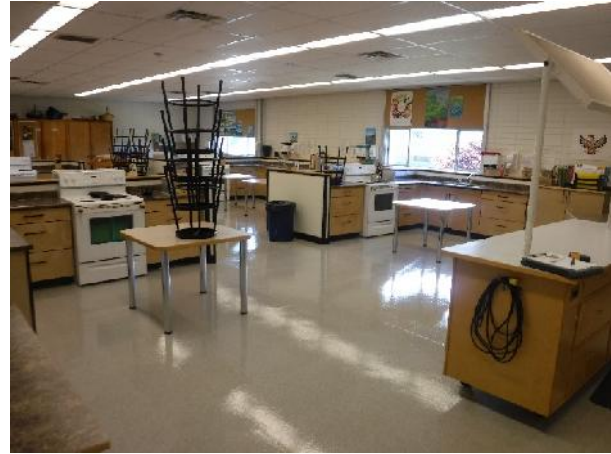
Photo 28 Description: Sheet flooring 14 – Grey swirl Location: Room 229 Asbestos: Suspect
