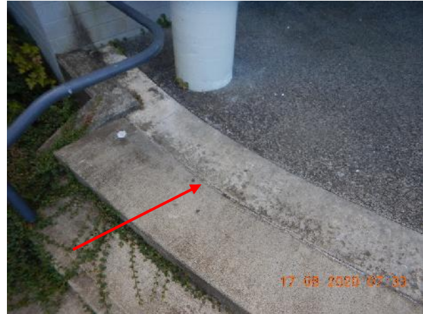
Photo 12 Description: Caulking 7 – Light Grey Location: Exterior Asbestos: Suspect concealed asbestos leveling compound(s)
