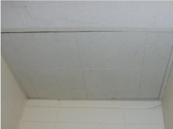
Photo 15 Description: Ceiling tile 1 – 12"x12" donnacona textured Location: Boys Change Room Asbestos: Suspect
