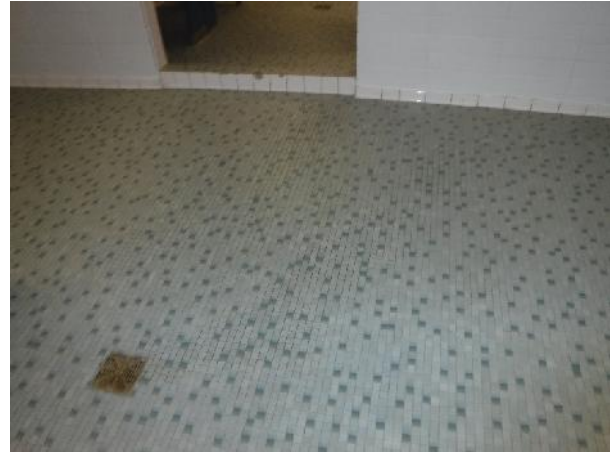
Photo 20 Description: 1"x1" green and grey ceramic tile grout and mortar Location: Girls Change Room Asbestos: Suspect
