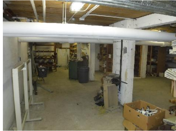
Photo 32 Description: Pipe run insulation Location: Basement Asbestos: Suspect
