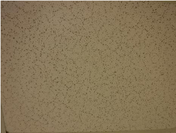
Photo 33 Description: Acoustic ceiling tile 1 – Patterned fissure small and large pinhole Location: Guys Instructor Asbestos: Suspect
