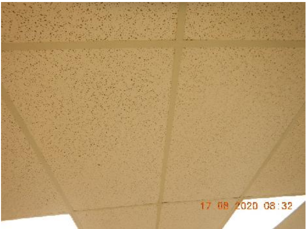
Photo 17 Description: Acoustic ceiling tile 4 – Random fissure, large pinholes Location: Room 100 Asbestos: Suspect
