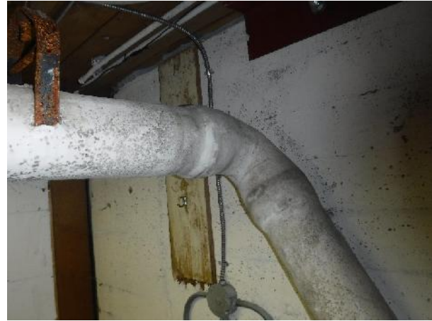
Photo 8 Description: Pipe elbow and fitting insulation Location: Basement Asbestos: 26% Chrysotile 4% Amosite Sample(s): 39957-9b,12b,13b
