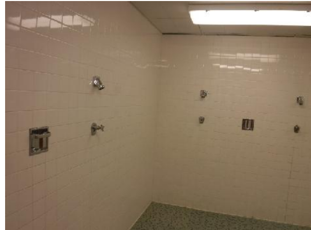
Photo 22 Description: 4"x4" white ceramic tile grout and mortar Location: Boys Change Room Asbestos: Suspect
