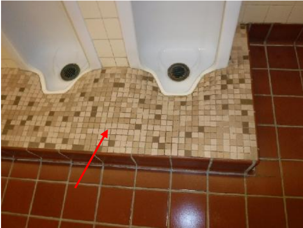
Photo 19 Description: 1"x1" beige and brown ceramic tile grout and mortar Location: Boys Washroom Off Hallway 3 Asbestos: Suspect
