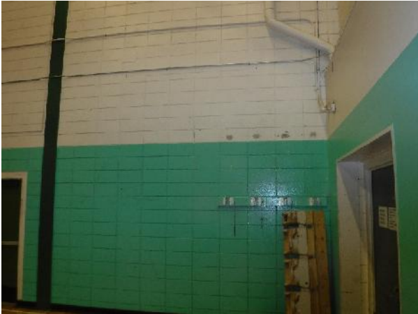
Photo 1 Description: Concrete block (contains vermiculite) Location: Gym Asbestos: 1% Actinolite Sample(s): 40391-48b
