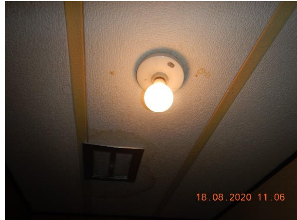
Photo 8 Description: Incandescent light gasket Location: Room 5 Asbestos: Suspect
