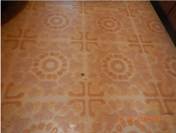
Photo 1 Description: Sheet flooring 9 – Yellow brown flower Location: Room 6 Asbestos: 20% Chrysotile Sample(s): 30008-2
