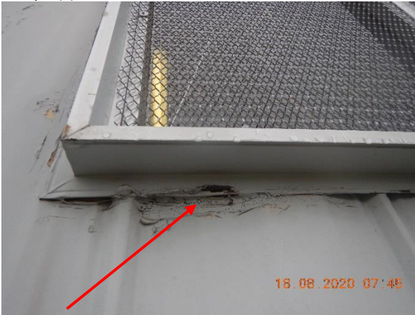
Photo 3 Description: Caulking 1 – Grey Location: Exterior Asbestos: Suspect
