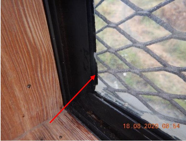
Photo 5 Description: Mastic 1 – Black Location: Room 1 Asbestos: Suspect
