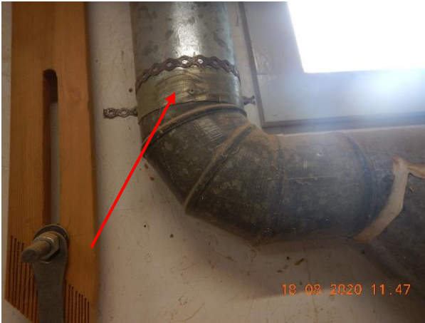
Photo 7 Description: Mastic 3 – Grey Location: Room 9 Asbestos: Suspect
