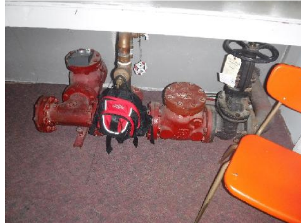
Photo 10 Description: Gaskets Location: Lower Storage Room N Asbestos: Suspect
