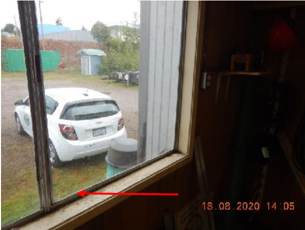
Photo 9 Description: Mastic type 2 – Black Location: Main Workshop Asbestos: Suspect
