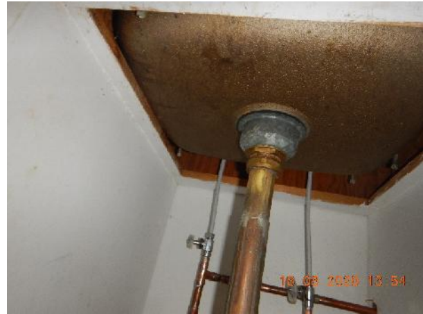
Photo 8 Description: Mastic type 1 – Gold/silver Location: Kitchen M Asbestos: Suspect
