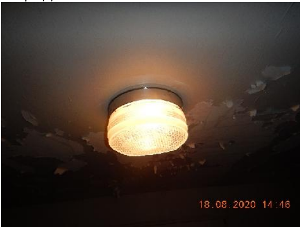
Photo 3 Description: Incandescent light gasket Location: Storage Room F Asbestos: 35% Chrysotile Sample(s): 30008-7
