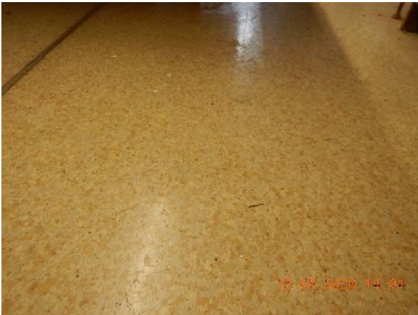
Photo 1 Description: Sheet flooring 11- Yellow/beige square mosaic Location: Main Workshop Asbestos: 20% Chrysotile Sample(s): 30008-4
