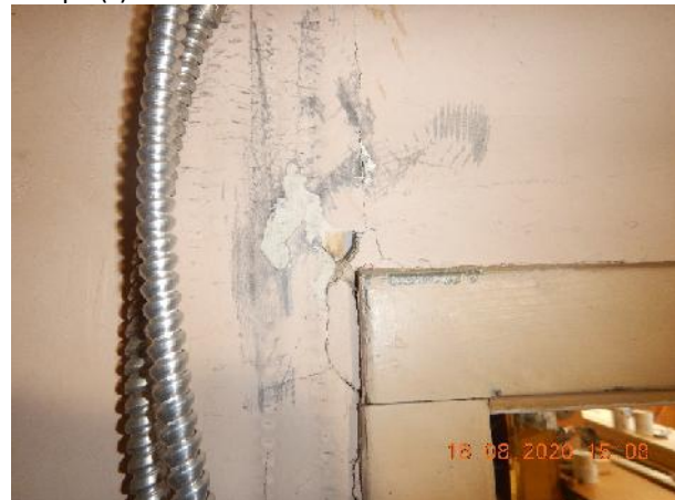
Photo 4 Description: Drywall with joint compound Location: Mechanical Room Asbestos: 1.5% Chrysotile Sample(s): 39957-24b
