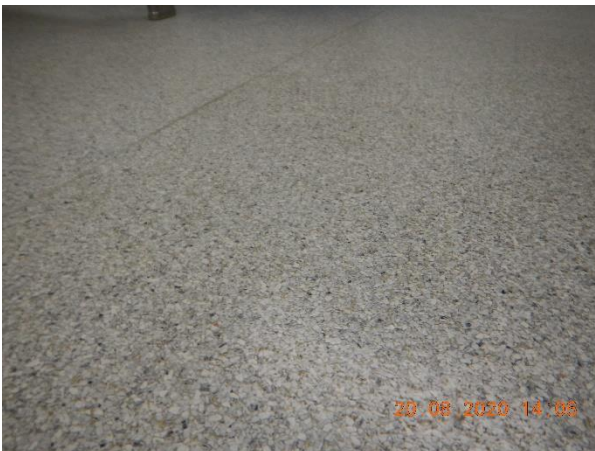
Photo 3 Description: Sheet flooring 1 – Light grey with black specks Location: Boys Washroom Asbestos: Suspect
