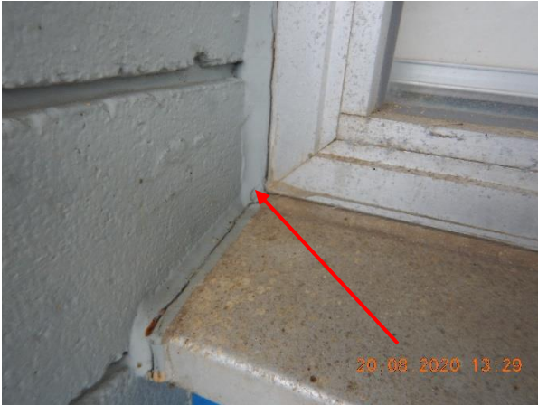
Photo 1 Description: Caulking – Grey Location: Exterior Asbestos: Suspect
