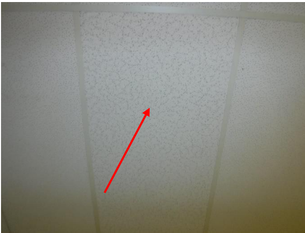
Photo 11 Description: Acoustic ceiling tile type 2 - Patterned fissures small and large pinhole Location: Office 2 Asbestos: Suspect
