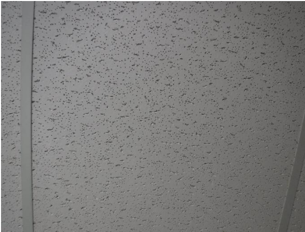
Photo 7 Description: Acoustic ceiling tile type 3 - Lateral fissures with pinholes
