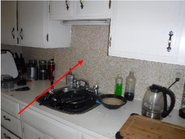
Photo 1 Description: Sheet flooring 1 – beige mosaic Location: Kitchen backsplash Asbestos: Suspect
