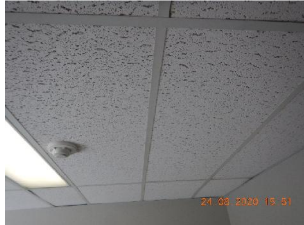
Photo 6 Description: Acoustic ceiling tile 1 – Vertical fissures and pinholes Location: 2nd Floor Admin Assistant Asbestos: Suspect concealed asbestos leveling compound(s)
