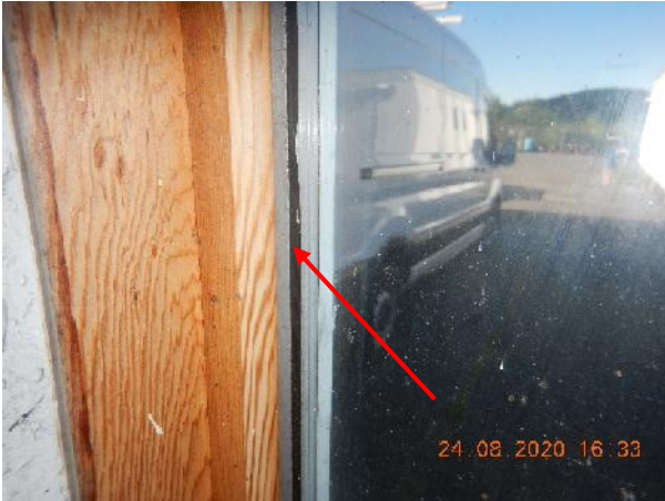
Photo 5 Description: Window Putty – Black Location: Carpentry Shop Asbestos: Suspect
