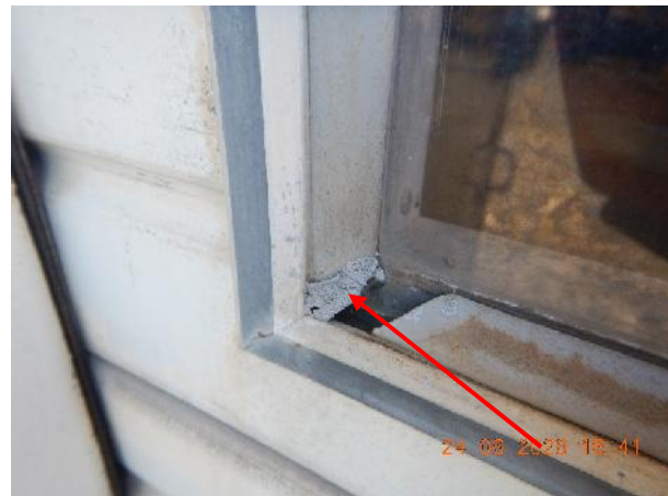
Photo 4 Description: Caulking – Grey Location: Exterior Garage Door Window Asbestos: Suspect
