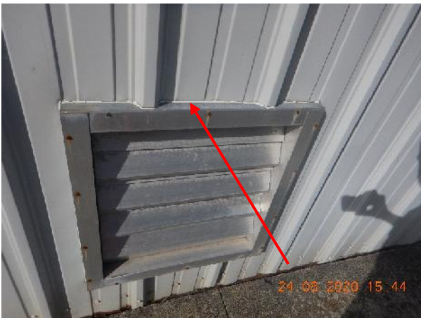
Photo 3 Description: Caulking – White Location: Exterior Asbestos: Suspect
