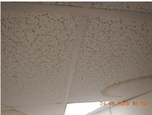
Photo 5 Description: Acoustic ceiling tile 2 – Patterned fissure small and large pinhole Location: 2 nd Floor Drafting Area Asbestos: Suspect
