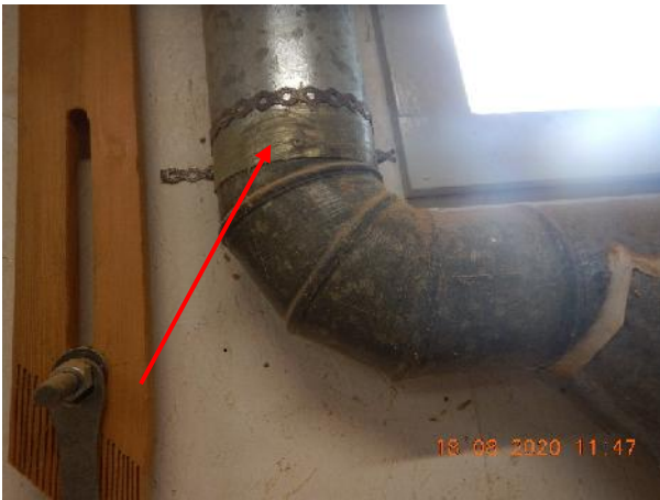
Photo 7 Description: Mastic 3 – Grey Location: Room 9 Asbestos: Suspect
