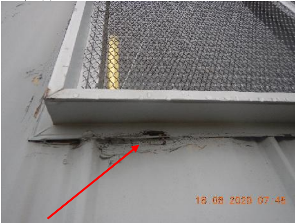
Photo 3 Description: Caulking 1 – Grey Location: Exterior Asbestos: Suspect
