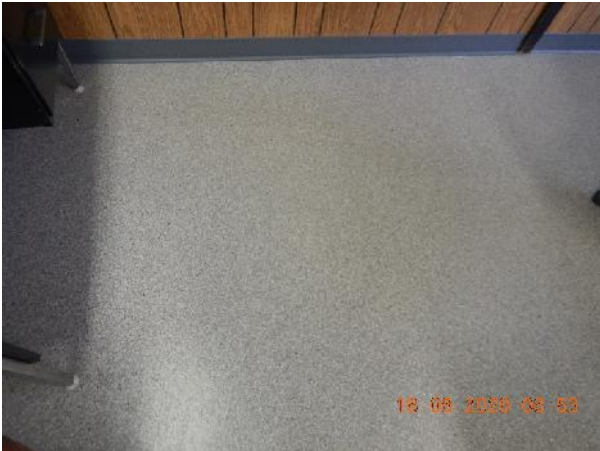
Photo 11 Description: Baseboard Adhesive
