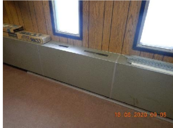
Photo 10 Description: Radiator (may contain concealed ACM insulation)
