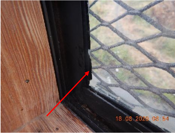
Photo 5 Description: Mastic 1 – Black Location: Room 1 Asbestos: Suspect
