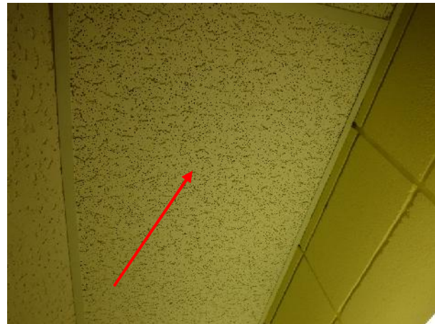
Photo 4 Description: Acoustic ceiling tile 4 – Horizontal fissure small pinhole Location: Boys Washroom Asbestos: Suspect
