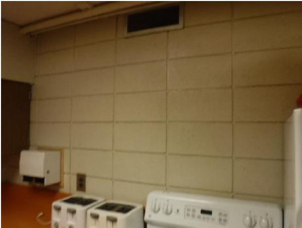
Photo 7 Description: Concrete blocks (may contain vermiculite) Location: Kitchen by Gym Asbestos: Suspect
