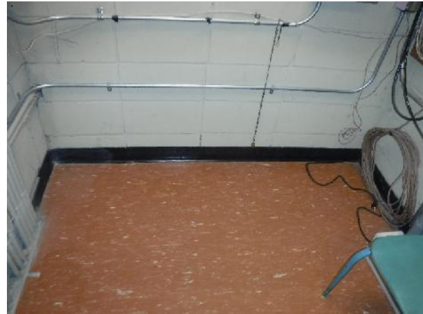
Photo 20 Description: Baseboard adhesive Location: Electrical Room Asbestos: Suspect
