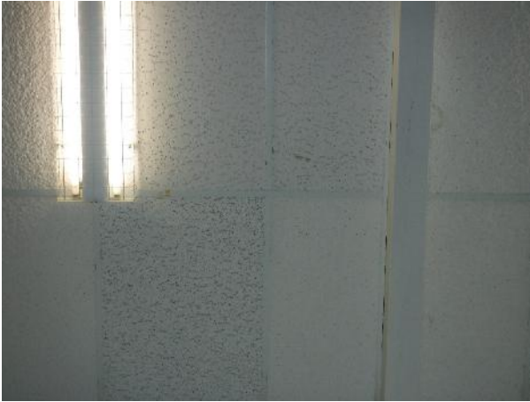
Photo 5 Description: Acoustic ceiling tile 5 – Textured 2'x4' Location: Gym Asbestos: Suspect
