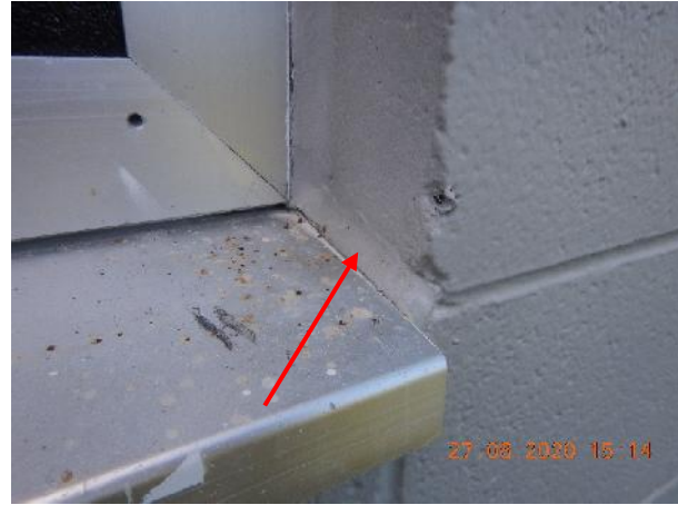
Photo 22 Description: Caulking 3 – Grey Location: Exterior Asbestos: Suspect
