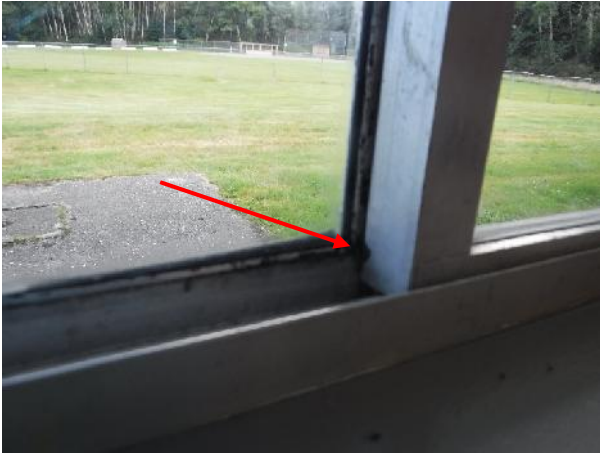
Photo 13 Description: Mastic 3 – Black Location: Community Rental B Asbestos: Suspect
