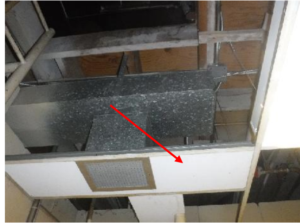
Photo 6 Description: Acoustic ceiling tile 6 – Textured ceiling tile Location: Janitor Room Asbestos: Suspect
