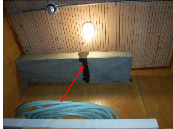
Photo 14 Description: Mastic 4 – Black Location: Community Rental A Janitor Asbestos: Suspect
