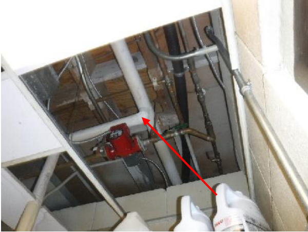
Photo 17 Description: Fittings insulation 1 - Cementitious Location: Janitor Room Asbestos: Suspect
