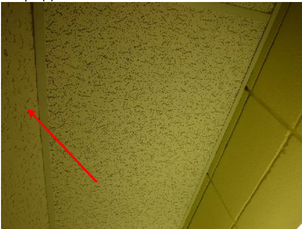
Photo 3 Description: Acoustic ceiling tile 3 – Longitudinal fissure small pinhole Location: Boys Washroom Asbestos: Suspect
