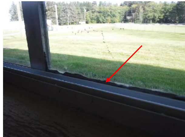
Photo 12 Description: Mastic 2 – Grey Location: Community Rental A Asbestos: Suspect
