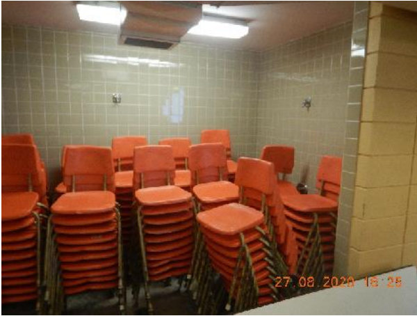
Photo 9 Description: 4"x4" ceramic tile grout and thinset Location: Room 109 Boys Changeroom Asbestos: Suspect concealed asbestos leveling compound(s)
