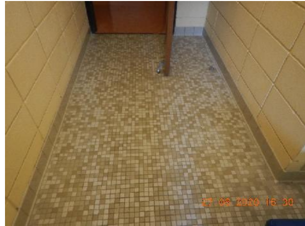
Photo 8 Description: 1"x1" ceramic tile grout and thinset Location: Room 110 Girls Changeroom Asbestos: Suspect concealed asbestos leveling compound(s)
