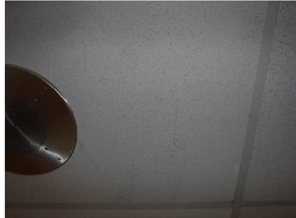
Photo 2 Description: Acoustic ceiling tile 1 – Small pinhole Location: Main Entry Hallway Asbestos: Suspect
