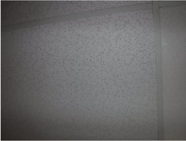
Photo 21 Description: Acoustic ceiling tile 2 – Patterned fissure small and large pinhole Location: Main Entry Hallway Asbestos: Suspect
