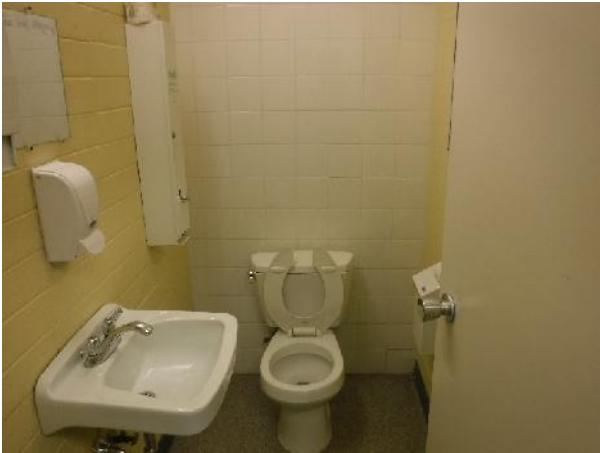
Photo 15 Description: White 6"x6" ceramic tile grout and thinset Location: Room 211 Asbestos: Suspect
