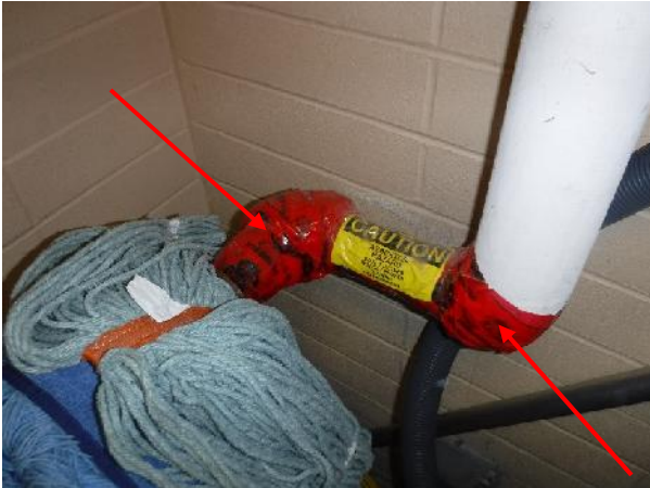
Photo 1 Description: Fittings insulation Location: Room 207 Asbestos: 40 % Chrysotile Sample(s): 30004-11
