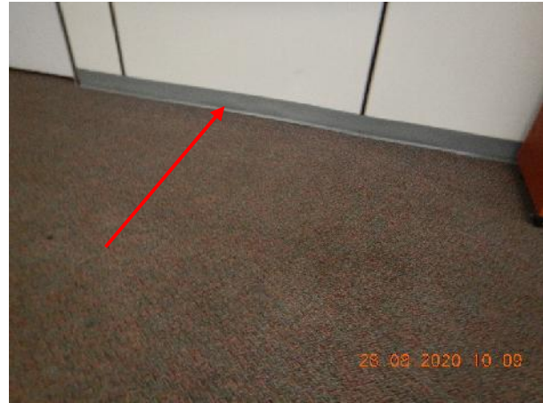
Photo 20 Description: Baseboard adhesive Location: Room 406 Asbestos: Suspect
