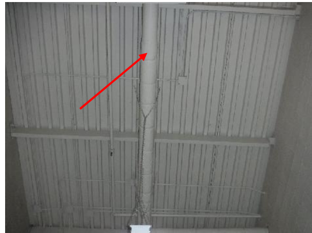
Photo 12 Description: Pipe run insulation Location: Room 310 Asbestos: Suspect
