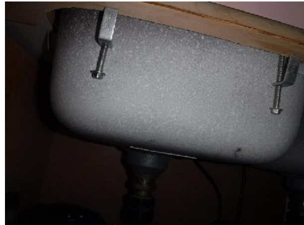
Photo 8 Description: Mastic – White Location: Room 303 sink Asbestos: Suspect
