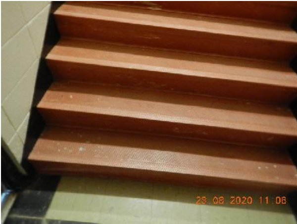
Photo 19 Description: Red stair tread Location: Room 314 stairwells Asbestos: Suspect
