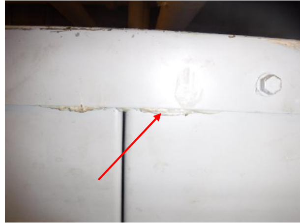
Photo 10 Description: Caulking type 1 – Grey Location: Room 307 mezzanine Asbestos: Suspect
