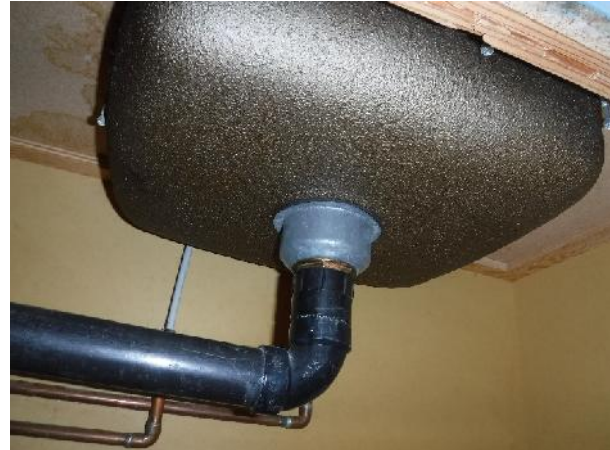
Photo 2 Description: Mastic – Silver/black Location: Room 204 Asbestos: 1.4% Chrysotile Sample(s): 30004-14
