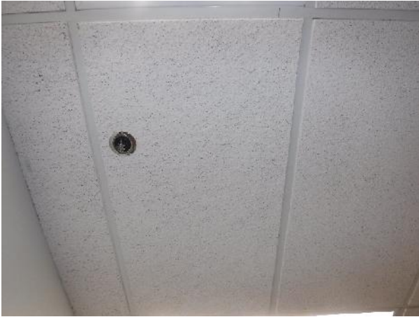
Photo 5 Description: Acoustic ceiling tile type 1 – Random fissure, dimpled, pinholes Location: Room 101 Asbestos: Suspect
