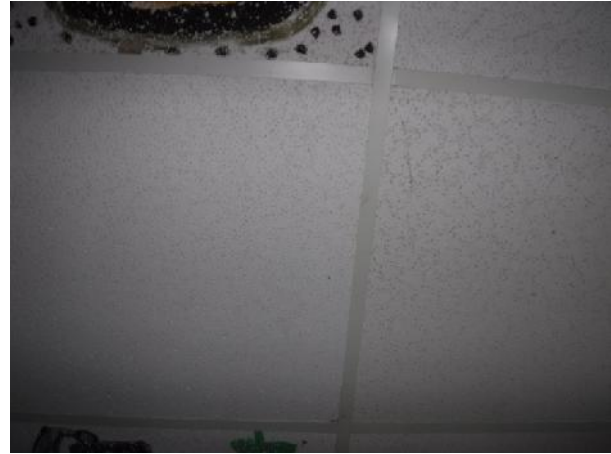
Photo 6 Description: Acoustic ceiling tile type 2 - Patterned fissures small and large pinhole Location: Hallway 4 Asbestos: Suspect
