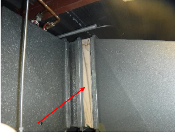
Photo 13 Description: Vibration dampeners Location: Room 307 mezzanine Asbestos: Suspect
