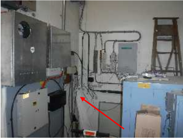
Photo 9 Description: Cement asbestos pipe
