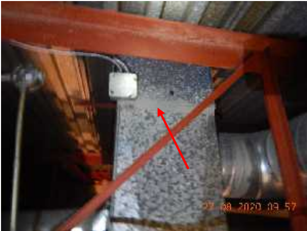
Photo 5 Description: Duct mastic – Grey Location: Janitor's Room Asbestos: Suspect
