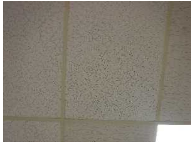
Photo 6 Description: Acoustic ceiling tile 1 – Patterned fissure small and large pinholes Location: Hallway Asbestos: Suspect
