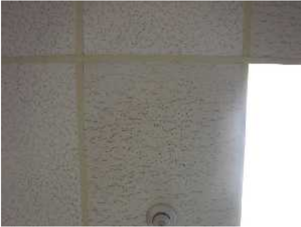
Photo 5 Description: Acoustic ceiling tile 2 – Lateral fissure Location: Hallway Asbestos: Suspect
