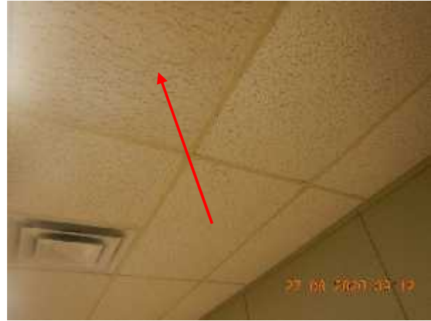
Photo 6 Description: Acoustic ceiling tile 3 – Vertical fissure Location: Room 2 Asbestos: Suspect
