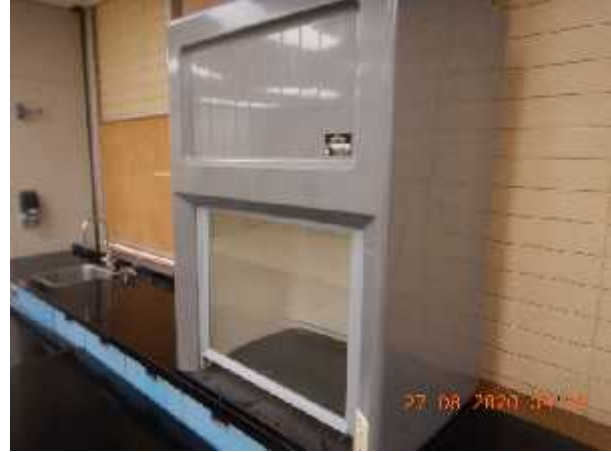
Photo 6 Description: Fume hood liner Location: Room 2 Asbestos: Suspect
