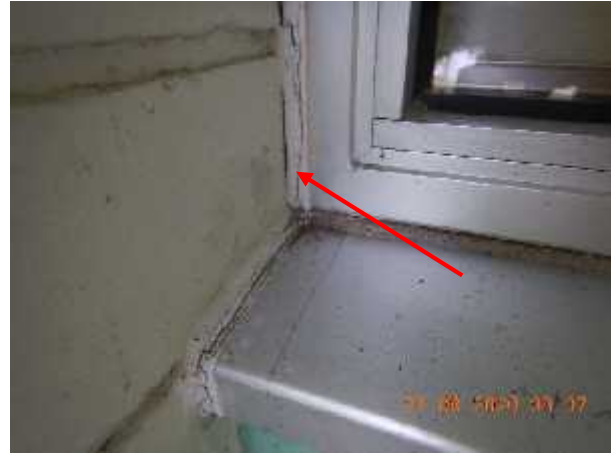
Photo 6 Description: Caulking type 1 – Grey Location: Exterior Asbestos: Suspect
