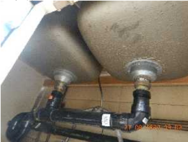
Photo 3 Description: Sink mastic – Gold Location: Room 4 (Home Economics) Asbestos: 1.9% Chrysotile Sample(s): 30710-6
