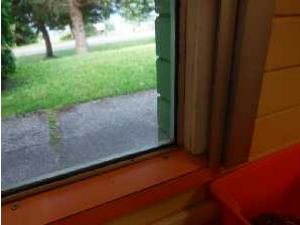
Photo 1 Description: Window putty (Black) Location: Thrift Store Asbestos: 12% Chrysotile Sample(s): 39957-51
