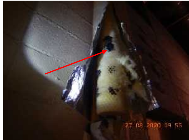
Photo 6 Description: Black mastic on fibreglass pipe insulation Location: Janitor's Room Asbestos: Suspect
