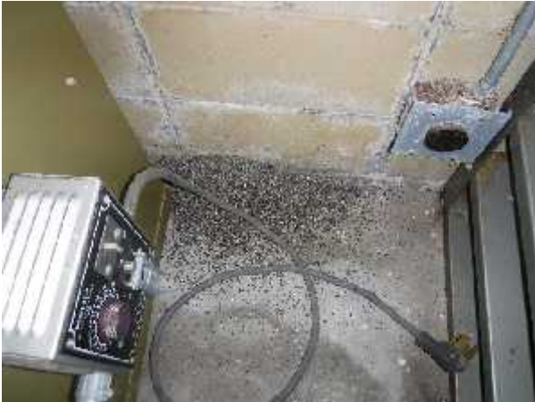
Photo 1 Description: Concrete block (contains vermiculite insulation) Location: Storage Room B Asbestos: 0.5% Actinolite Sample(s): 39957-53b
