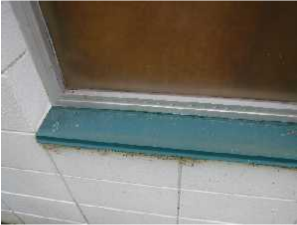
Photo 5 Description: Caulking 1 – Grey Location: Exterior Asbestos: Suspect
