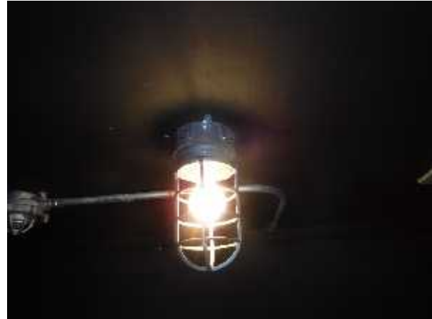
Photo 2 Description: Gasket 1 Location: Dark Room Asbestos: Suspect
