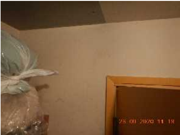
Photo 1 Description: Drywall with joint compound Location: Store Room Asbestos: 1.4%-3.9% Chrysotile Sample(s): 30010-7, 9, 10, 11, 13
