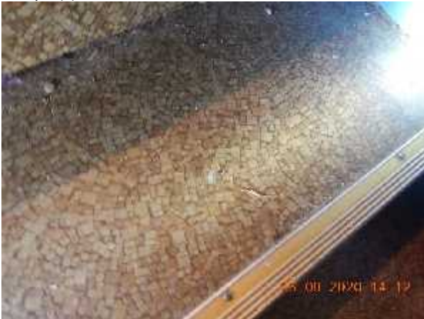
Photo 3 Description: Sheet flooring 5 – Beige red mosaic Location: Gym Stage Stairs Asbestos: 7.1% Chrysotile Sample(s): 30010-25
