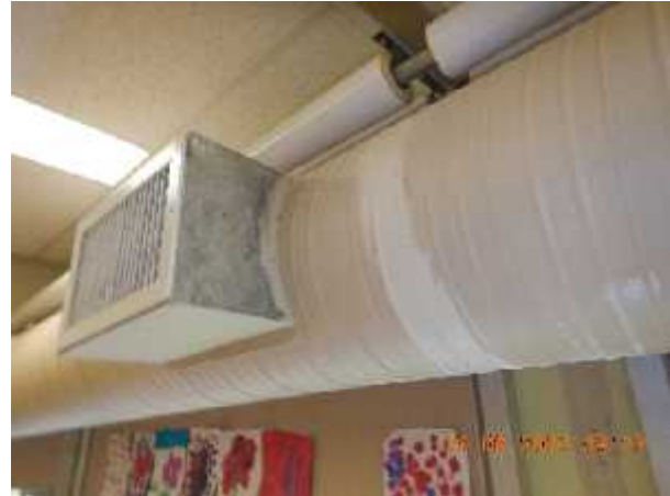
Photo 18 Description: Mastic 1- Grey (painted white in some locations) Location: Classroom D Asbestos: Suspect
