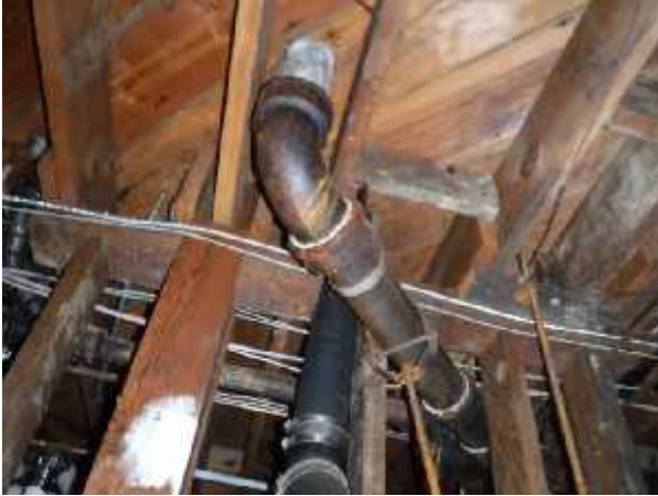
Photo 25 Description: Bell and spigot pipe gaskets Location: Crawl Space Asbestos: Suspect
