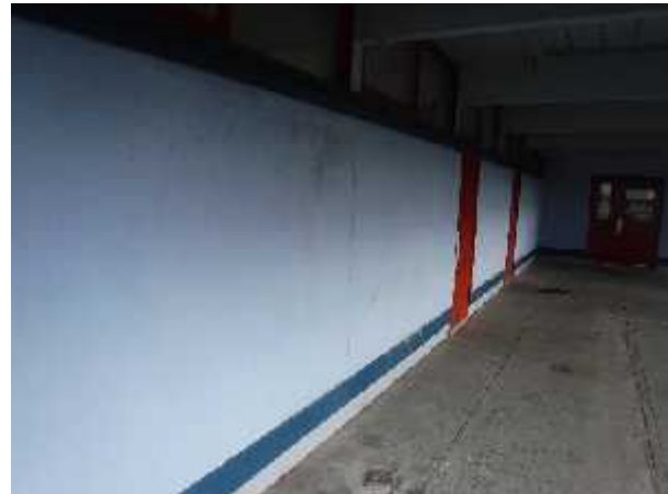
Photo 8 Description: Stucco Location: Exterior Asbestos: Suspect
