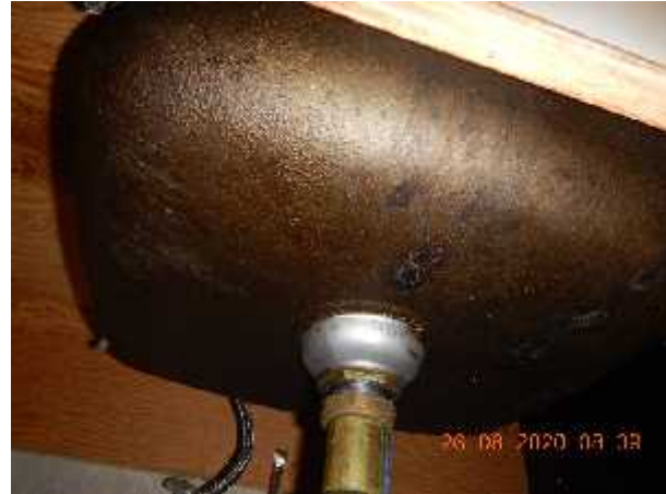
Photo 6 Description: Caulking – Acoustical sink insulation (Black) Location: Classroom 2 Sink Asbestos: 2.5% Chrysotile Sample(s): 30010-6
