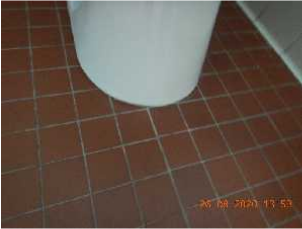
Photo 13 Description: Ceramic tile 2 – 2"x2" brown Location: Men's Washroom Asbestos: Suspect concealed asbestos leveling compound(s)
