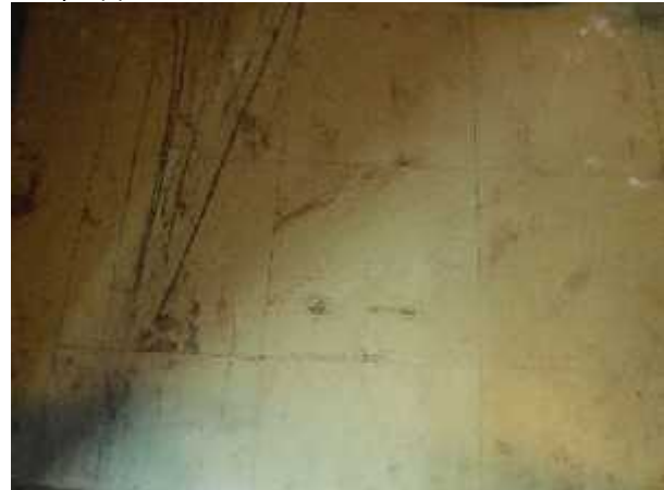
Photo 4 Description: Floor tile 2 – 9”x9” Beige Location: Gym Mechanical Room Asbestos: 3.1% Chrysotile Sample(s): 30010-24
