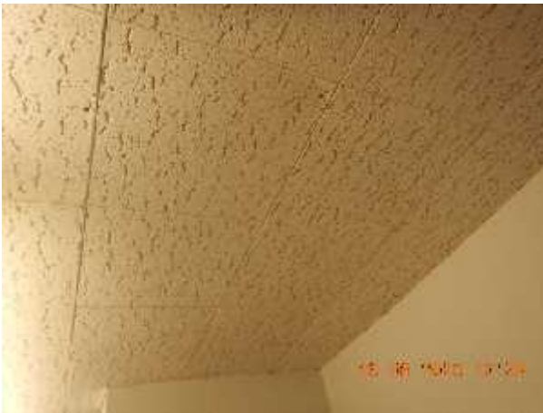
Photo 15 Description: Acoustic ceiling tile 3 – 12"x12" vertical fissure small and large pinhole Location: Main Office Asbestos: Suspect
