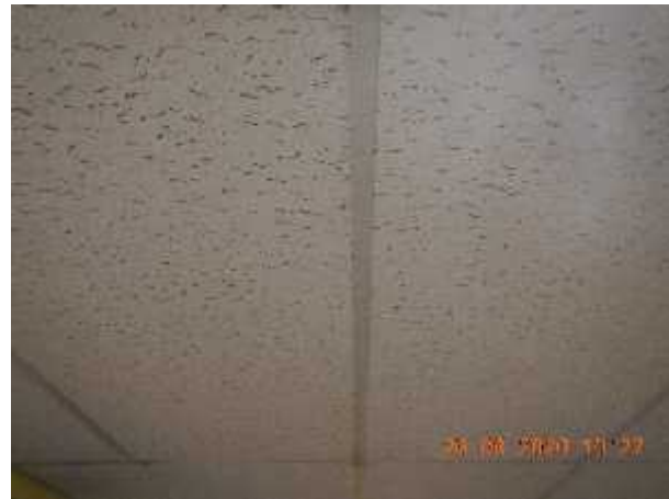
Photo 16 Description: Acoustic ceiling tile 5 – 2'x4' lateral fissure small and large pinhole Location: Basement Classroom Corridor Asbestos: Suspect
