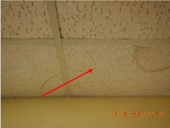
Photo 17 Description: Acoustic ceiling tile 6 – 2'x4' small and large pinhole Location: Basement Classroom Corridor Asbestos: Suspect
