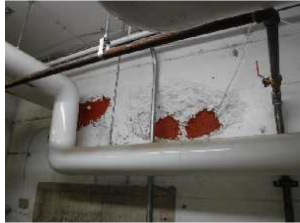
Photo 22 Description: Penetration caulking – Red Location: Boiler/Hot Water Room Asbestos: Suspect
