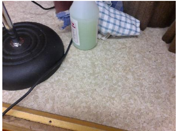
Photo 2 Description: Sheet flooring – SF8 Medium Beige Mosaic Location: Gymnasium Asbestos: None detected Sample(s): 30002-16
