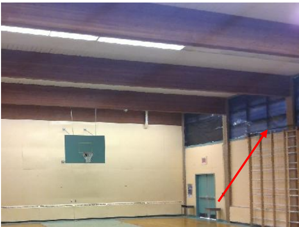
Photo 3 Description: Window putty Location: Gymnasium Asbestos: Suspect Sample(s): None
