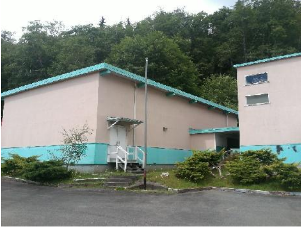
Photo 5 Description: Stucco Location: Exterior Hazmat: Contains crystalline silica and suspected to contain asbestos Sample(s): None
