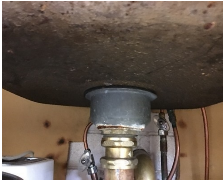
Mastic - Black/Brown on Sink (contains 3.2% Chrysotile asbestos)
